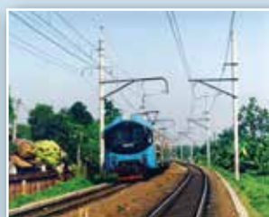
Railway Catenary Poles
